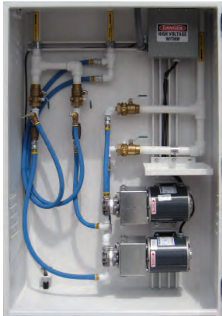
SPS-25-SD Mechanical Compartment
