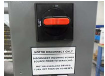
Motor Disconnect Switch
