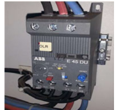
Overload Relay (OLR)
