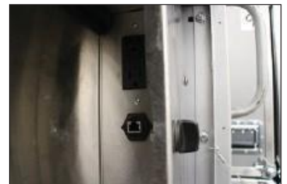
Figure 8: Load Bank HMI Connection
