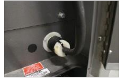
Figure 3: Fan/control Power Receptacle
